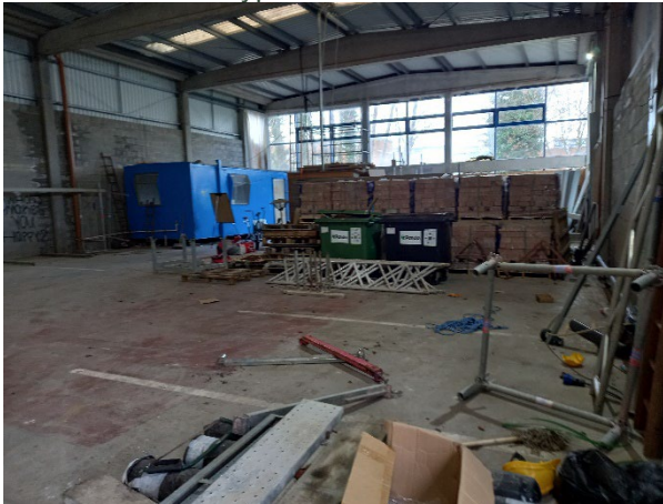
A3. Interior of building at the southwestern border of the site showing high light ingress.
